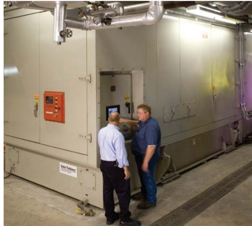
15 MW gas turbine generator set at Michigan State Univ., Solar Turbines Inc.
