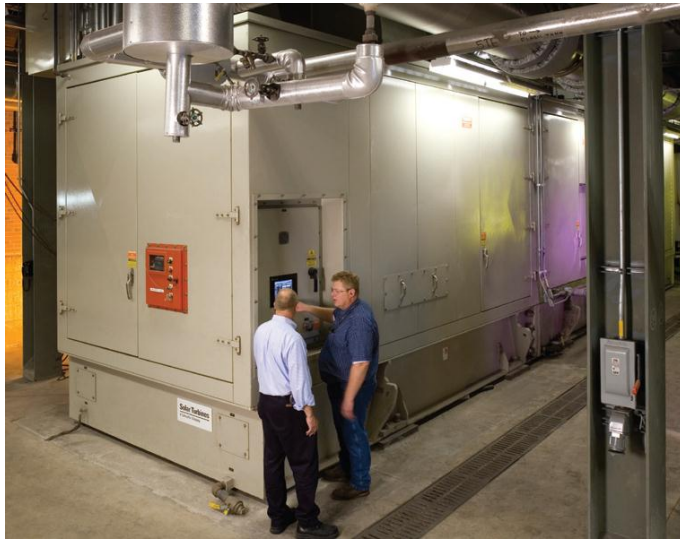
15 MW gas turbine generator set at Michigan State Univ., Solar Turbines Inc.
